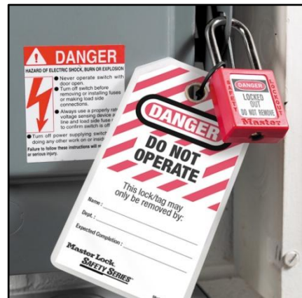
Switch with lock and red danger tag.
