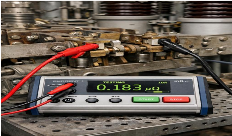
Fig.3.3.9.a. Micro-ohmmeter connected across breaker or tap changer contacts.
