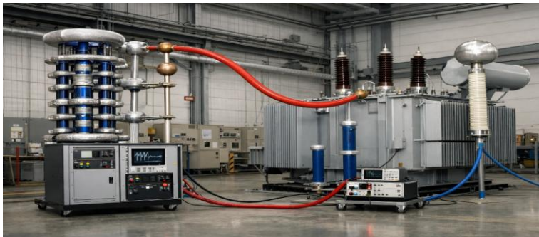
Fig.3.2.a. Factory testing setup with high-voltage impulse generator connected to transformer.
