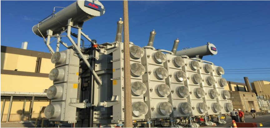
Fig.2.3.b Onsite Power Transformer with colling arrangement
