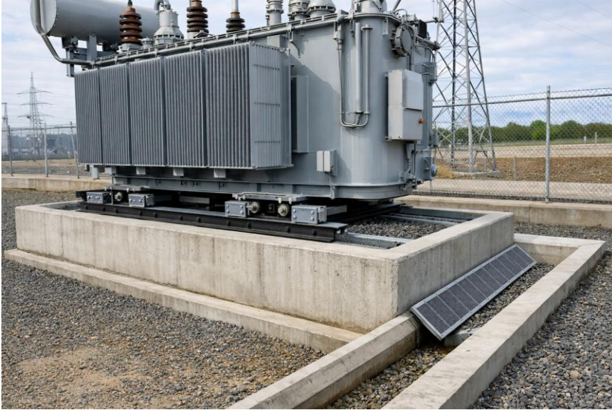
Fig.2.1.A.Side view showing transformer mounted on concrete foundation with rollers, plinth, and oil drain channel
