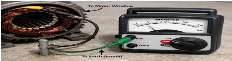
Fig.3.2.c.Megger connected between winding and earth.
